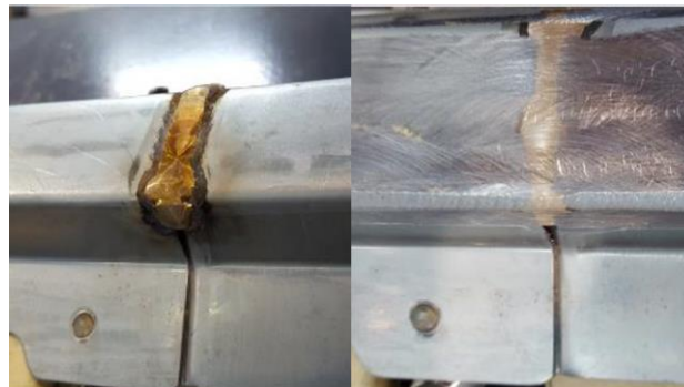
Figure 11. Welding beam. Left: Before being polished. Right: Welding beam after being polished.
